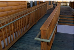
Fig 4-B. Curb Ramp at Accessible Parking
